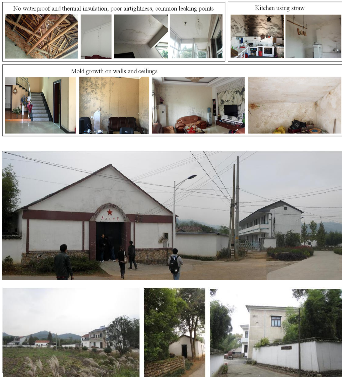
Fig. 2-13. Problems observed in rural houses during inspections
